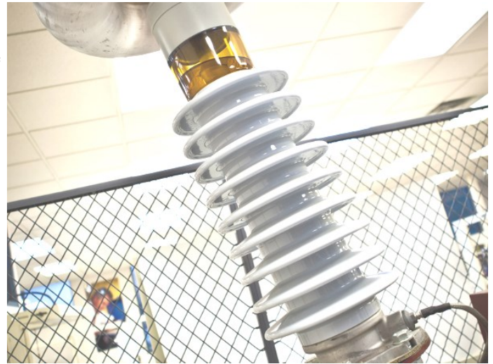
ELTEK's 150,000 VAC "Big Phenix" Transformer
